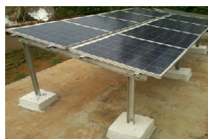
1 kW Photovoltaic Power Plant
